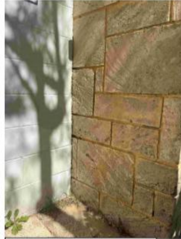
66 Main Building - West facade - Fretting mortar
