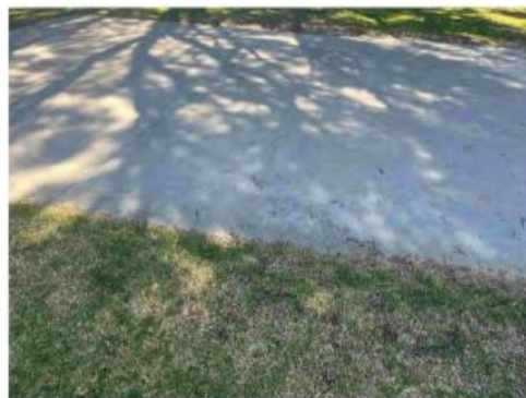
52 Concrete practice wall - Minor cracking
