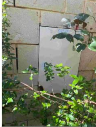
68 Main Building - South facade - Fretting mortar and switchboard corrosion
