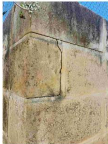
3 Retaining wall SW Minor damage
