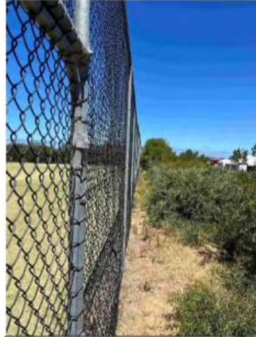
13 Northern boundary fence - Minor rotation
