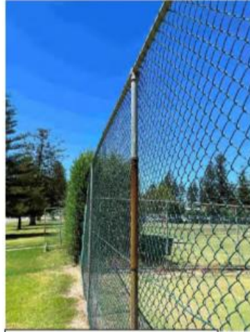
17 Eastern boundary fence - Minor rotation and rust
