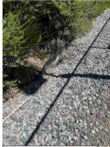
5 Western boundary fence Damaged drainage
