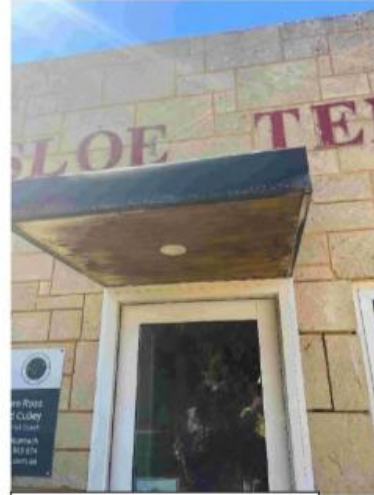
69 Main Building - South facade - Awning soffit damage
