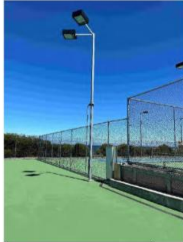
32 Hard court lighting and Power DB
