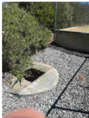
7 Western boundary fence - Old drainage grate
