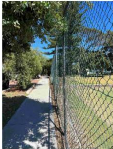
23 Southern boundary fence - Minor fence rotation
