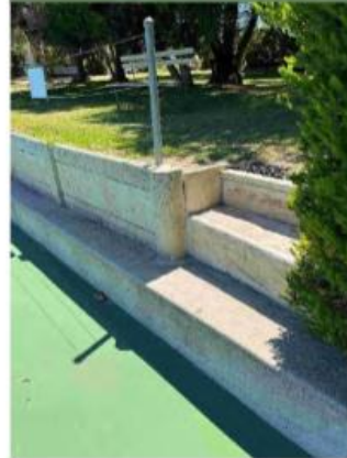
31 Hard court retaining Minor damage 1
