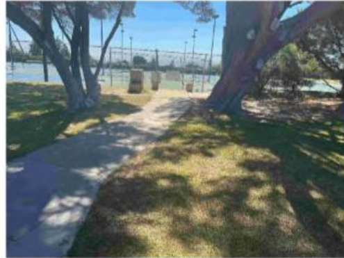
59 Internal concrete paths - damaged path
