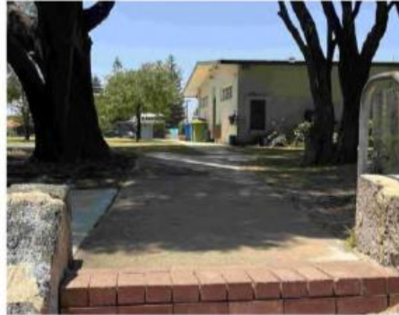
41 Internal concrete paths and stairs - damaged path
