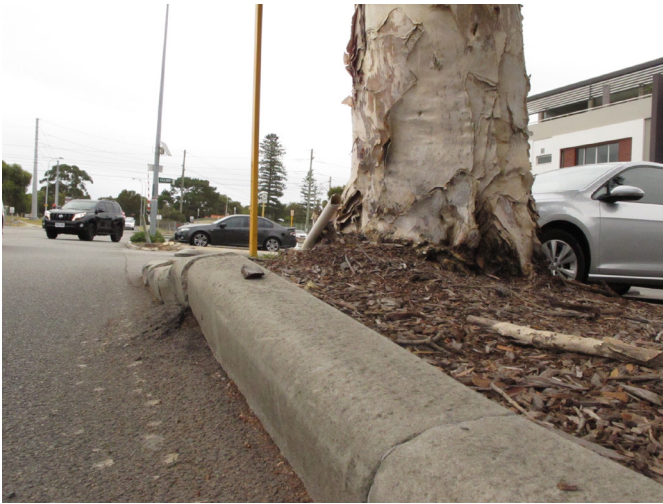
Figure 2: Melaleuca quinquenervia causing damage to road and curbing on Jarrad St.
