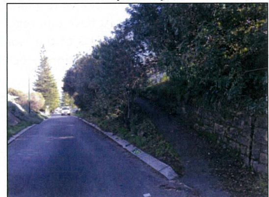
Figure 6 – Photo looking west along Deane Street demonstrating the embankment commencing at the edge of the carriageway.
