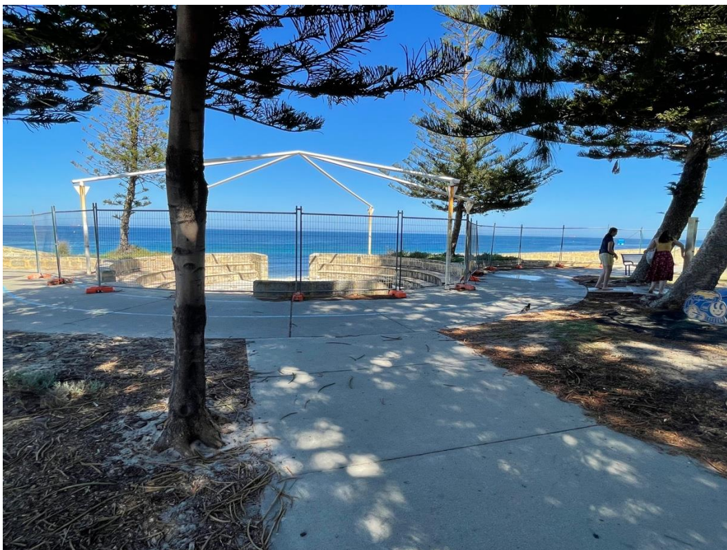
Photograph 14: All of this area will be renewed and the 1980s and 1990s structures removed Griffiths Architects January 2021.
