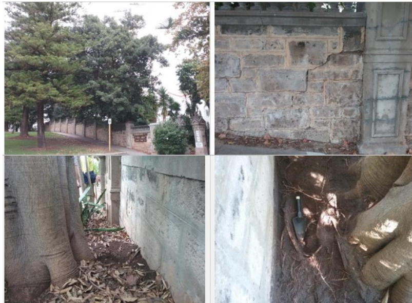
Figure 2: Tree roots damaging boundary wall
