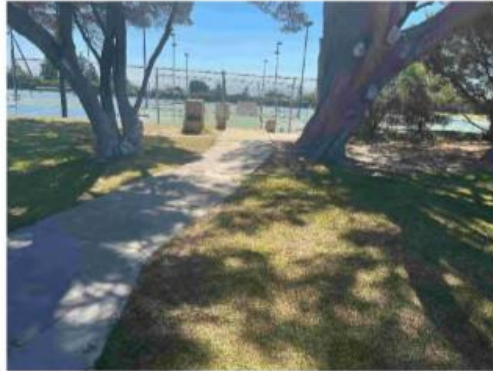
59 Internal concrete paths - damaged path
