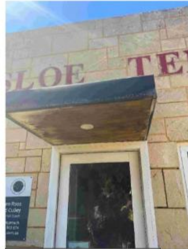
69 Main Building - South facade - Awning soffit damage
