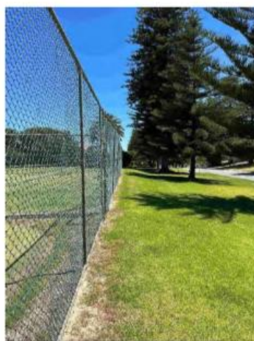
16 Eastern boundary fence - Minor rotation
