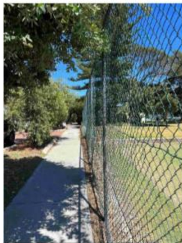
23 Southern boundary fence - Minor fence rotation
