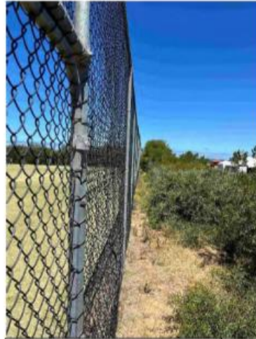
13 Northern boundary fence - Minor rotation
