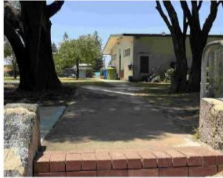
41 Internal concrete paths and stairs - damaged path
