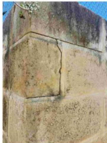
3 Retaining wall SW Minor damage
