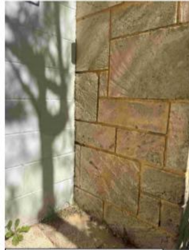
66 Main Building - West facade - Fretting mortar
