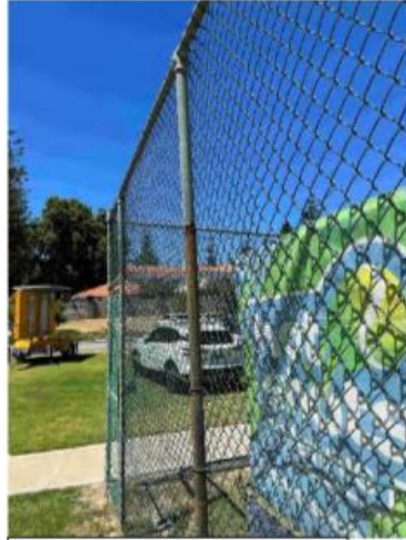
21 Eastern boundary fence - Minor rotation and rust
