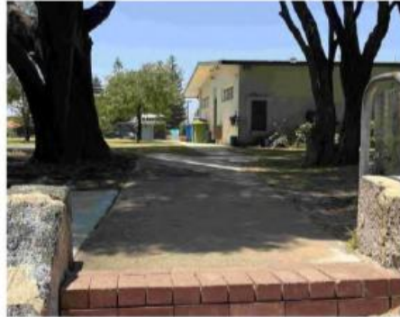
41 Internal concrete paths and stairs - damaged path
