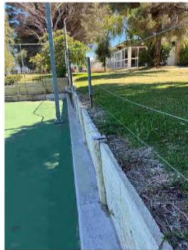
31a Hard court retaining Minor damage2
