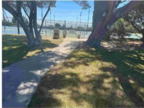
59 Internal concrete paths - damaged path
