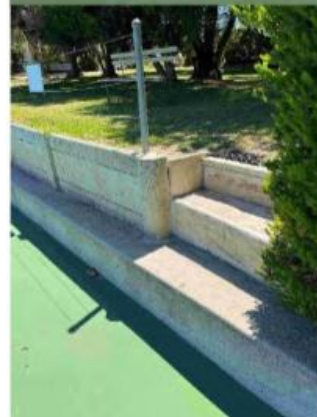
31 Hard court retaining Minor damage 1
