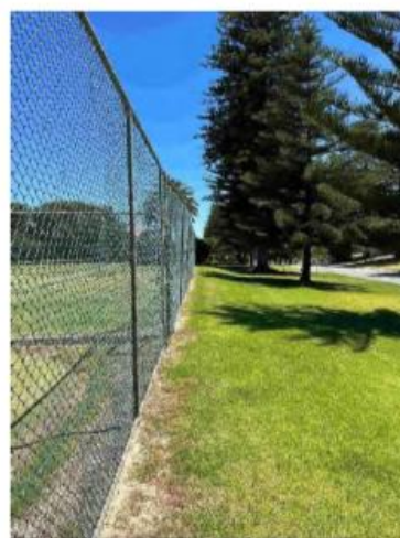
16 Eastern boundary fence - Minor rotation
