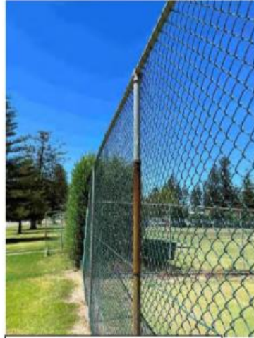
17 Eastern boundary fence - Minor rotation and rust
