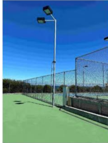
32 Hard court lighting and Power DB
