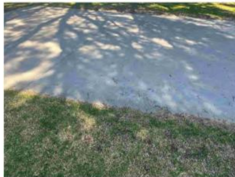
52 Concrete practice wall - Minor cracking
