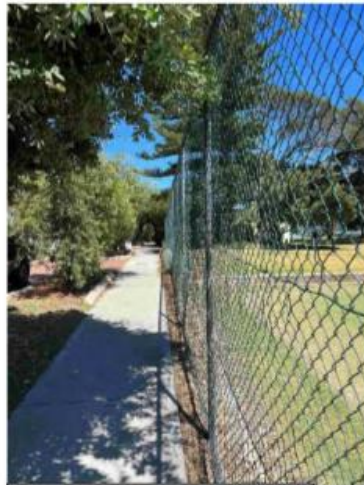
23 Southern boundary fence - Minor fence rotation
