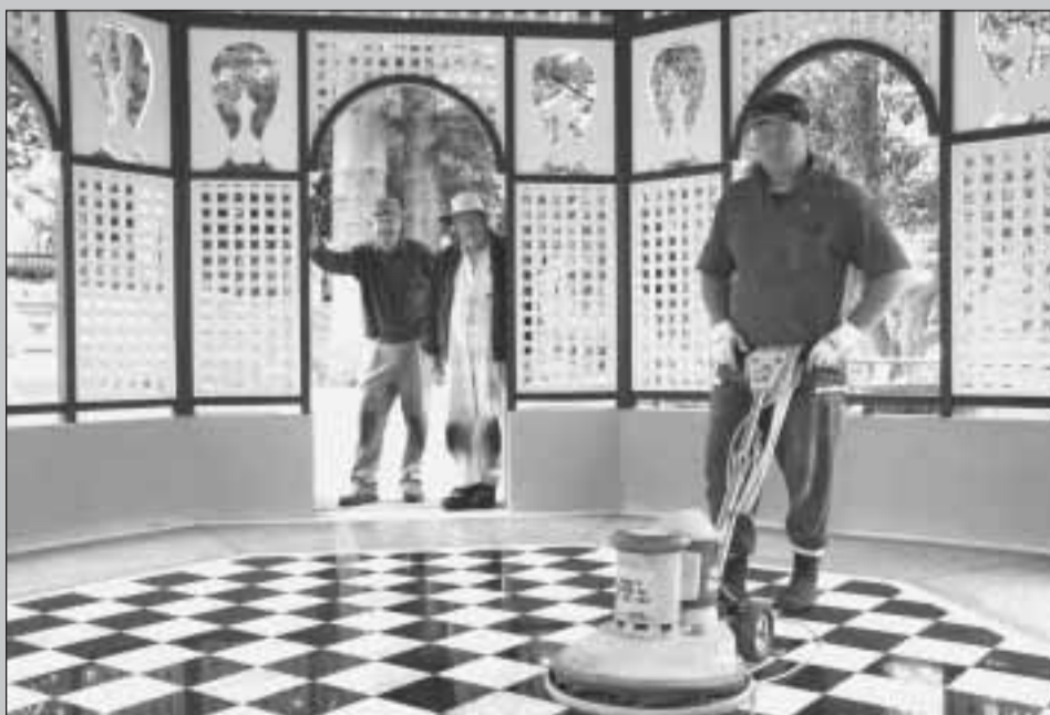
Finishing touches: Stonemason Andrew Furr polishes the century-old marble tiles, preserved from the original Summer House. In the doorway - conservator Ken Miller, driver and designer of the centenary project, with master craftsman Frank Warren.
