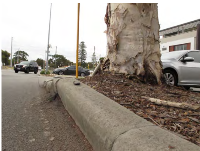
Figure 2: Melaleuca quinquenervia causing damage to road and curbing on Jarrad St.
